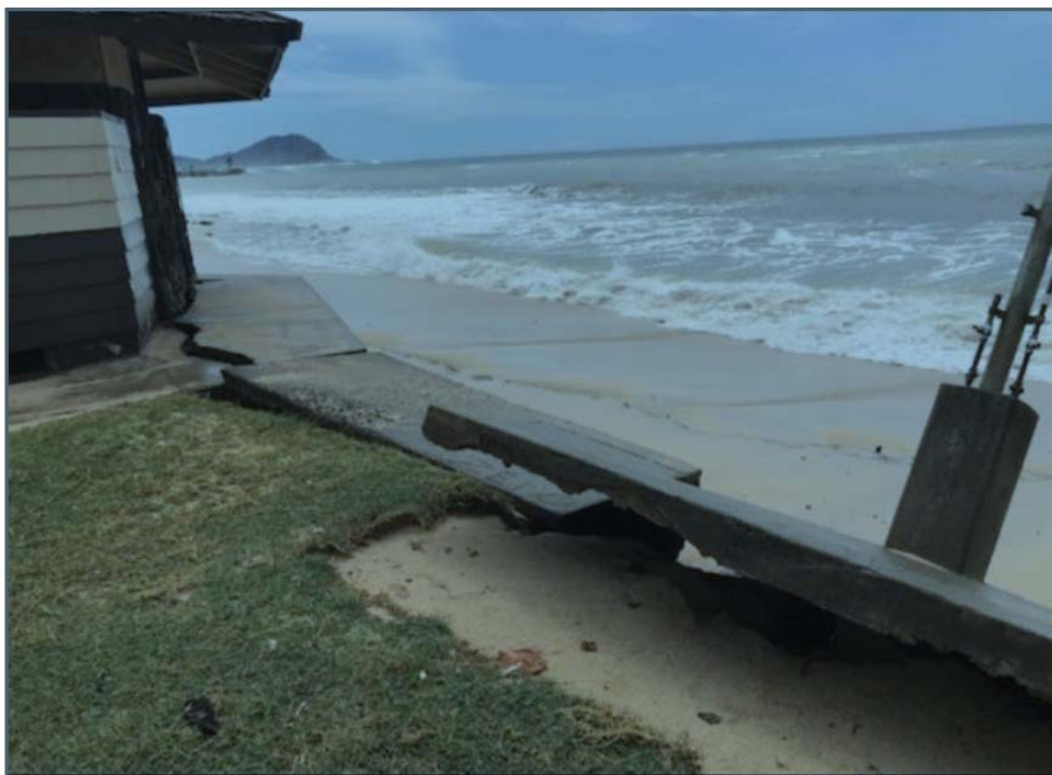
Figure 10: Destruction of Public Facilities, Maunalahilahi Beach Park, 2018
