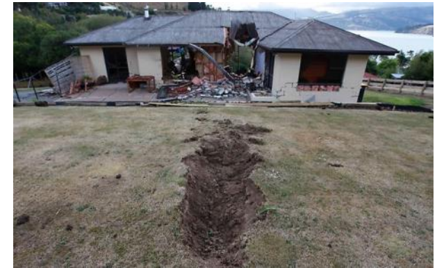
New Zealand Earthquake
